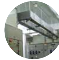
Low-voltage DC busbars
