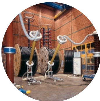
High voltage laboratory, partial discharge measurement and ac voltage test
